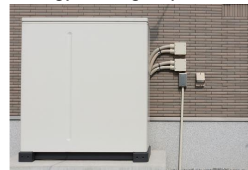
Energy storage system
