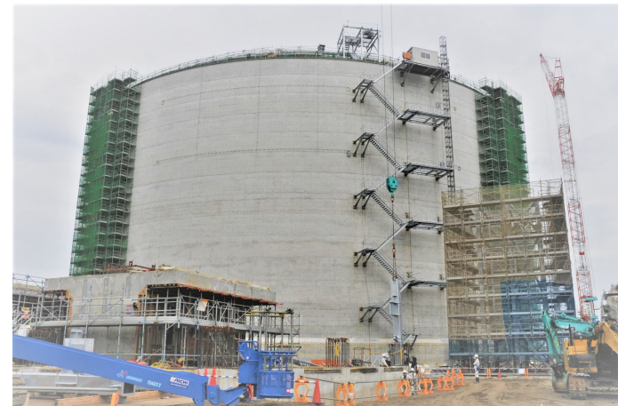
Building a LNG tank, the largest of its kind in Japan, on the premises of Ehime Works
